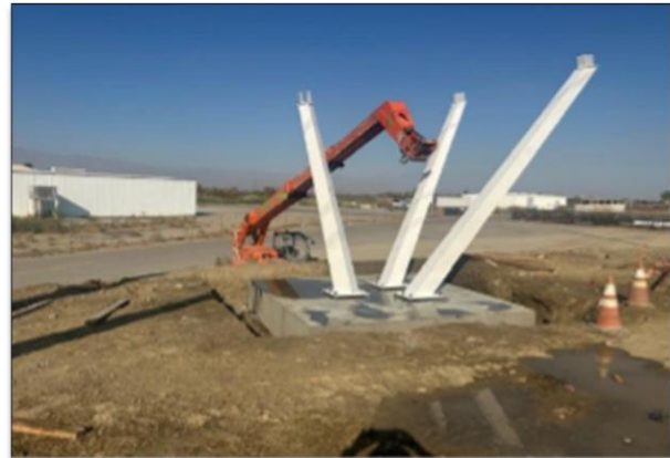
Install of shade structure columns at Airport North Access Point in Coachella
