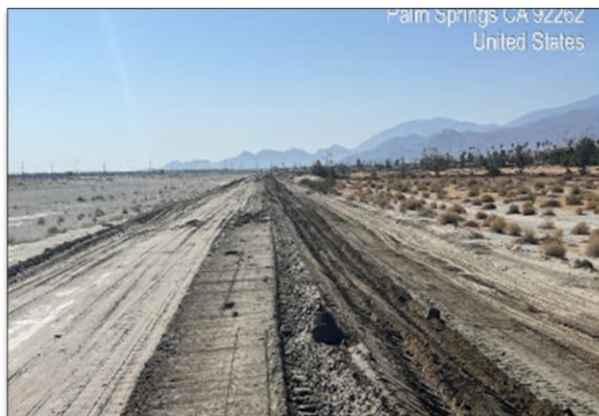
Grading and compacting for Jointed Plain Concrete Paving; N. Palm Canyon to Gene Autry.
