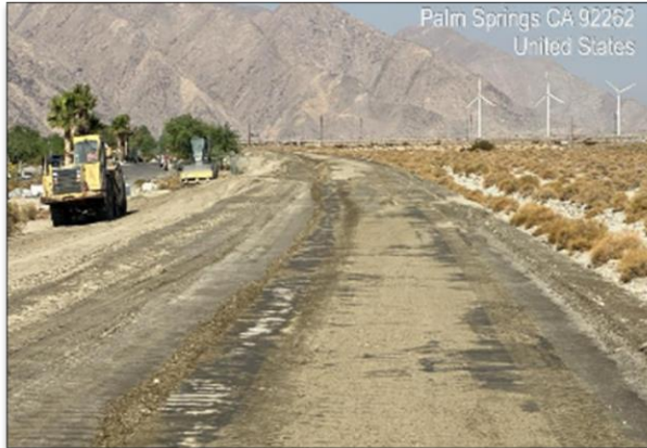
Grading dry side slopes for pathway realignment and grading and compacting for Jointed Plain Concrete Pavement; Sunrise Way to Gene Autry in Palm Springs..
