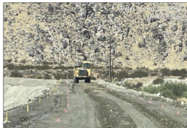
Grading and compacting from N. Palm Canyon to Gene Autry in Palm Springs.
