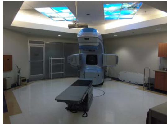
LINEAR ACCELERATOR IN VAULT
