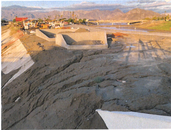
Existing Road at Ave 44 washed away
