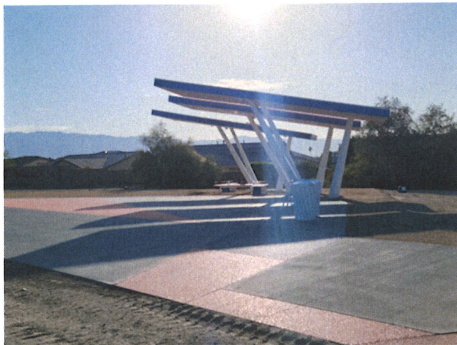
American Channel Access Point accessories installed.
